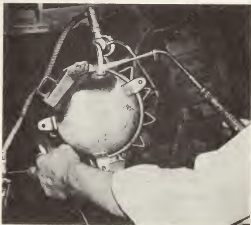
2-22. Silver brazing copper tubing to a compressor dome. Note carbon dioxide connection. (Handy & Harman)
